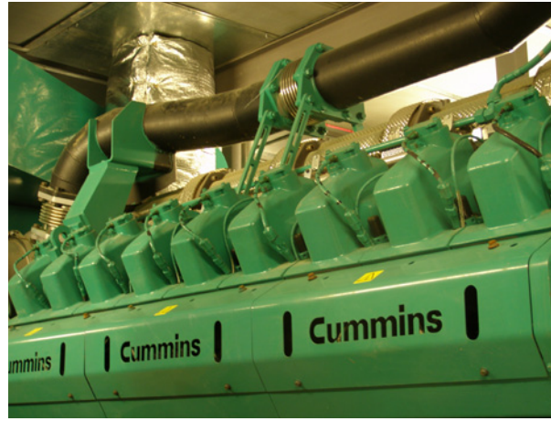
Cummins QSV91 lean-burn gas engines power the project
